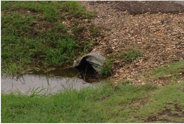
Figure 7C: Damaged Culvert Example
